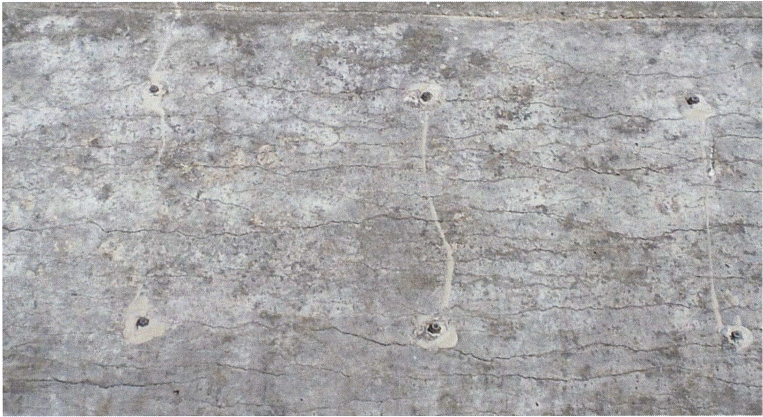
Figure 3-15. Longitudinal Cracks from ASR Expansion.
