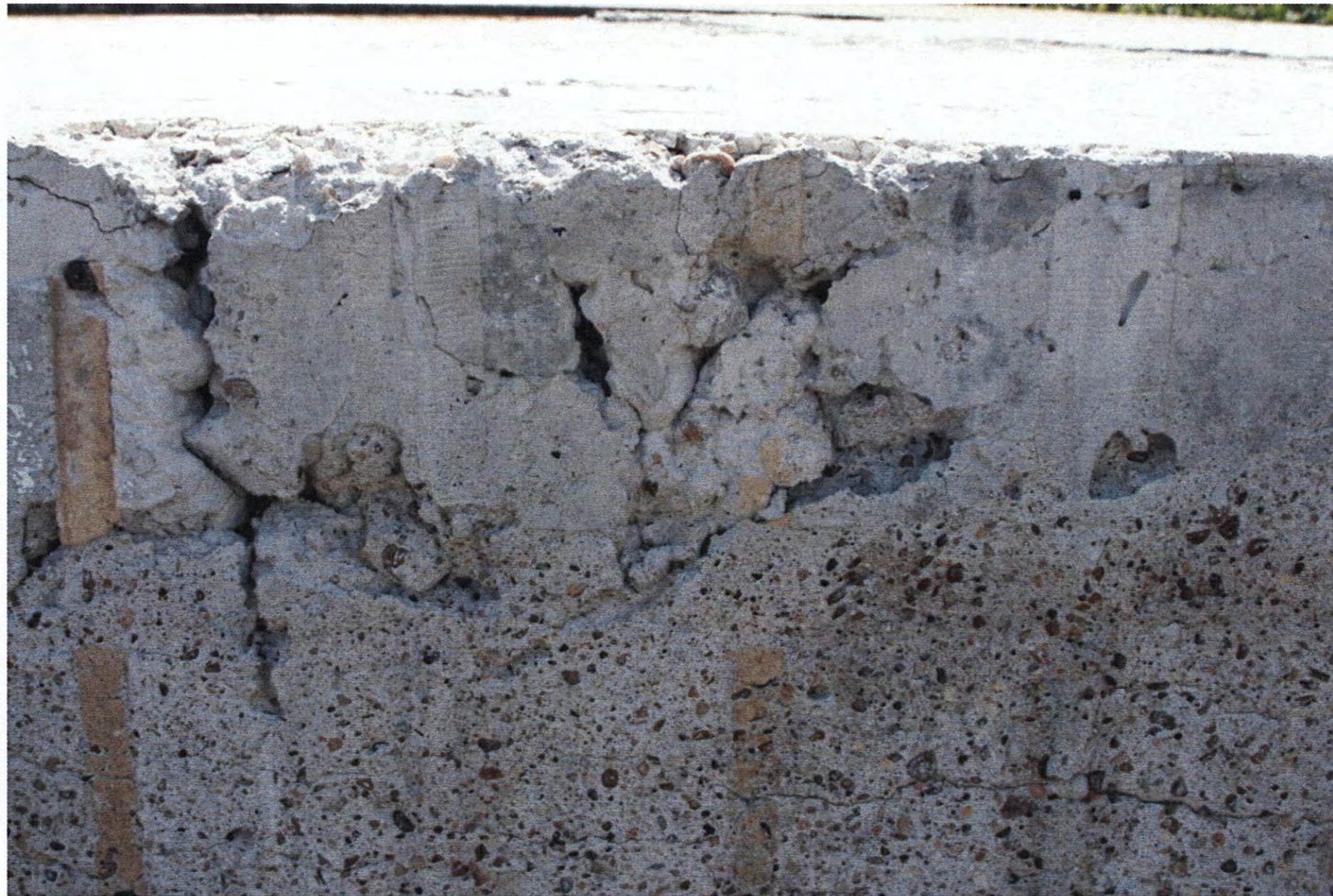
Figure 2-11. Voids in the First Trials.
