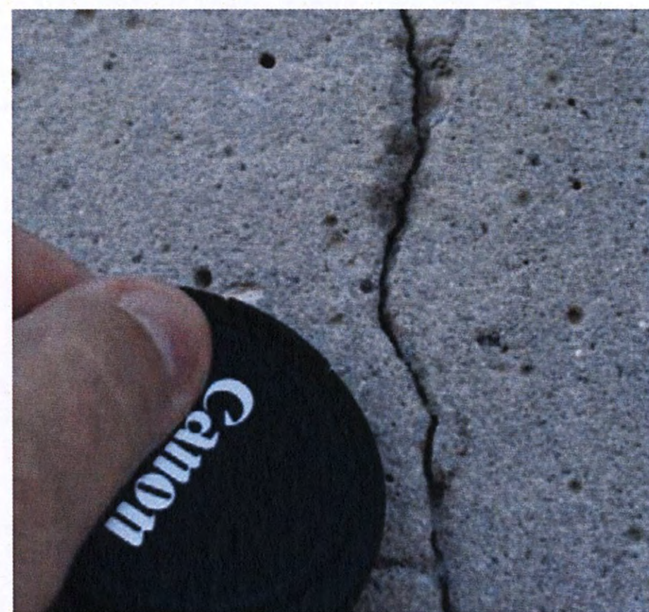
(b) Close-up View of a Typical Crack
