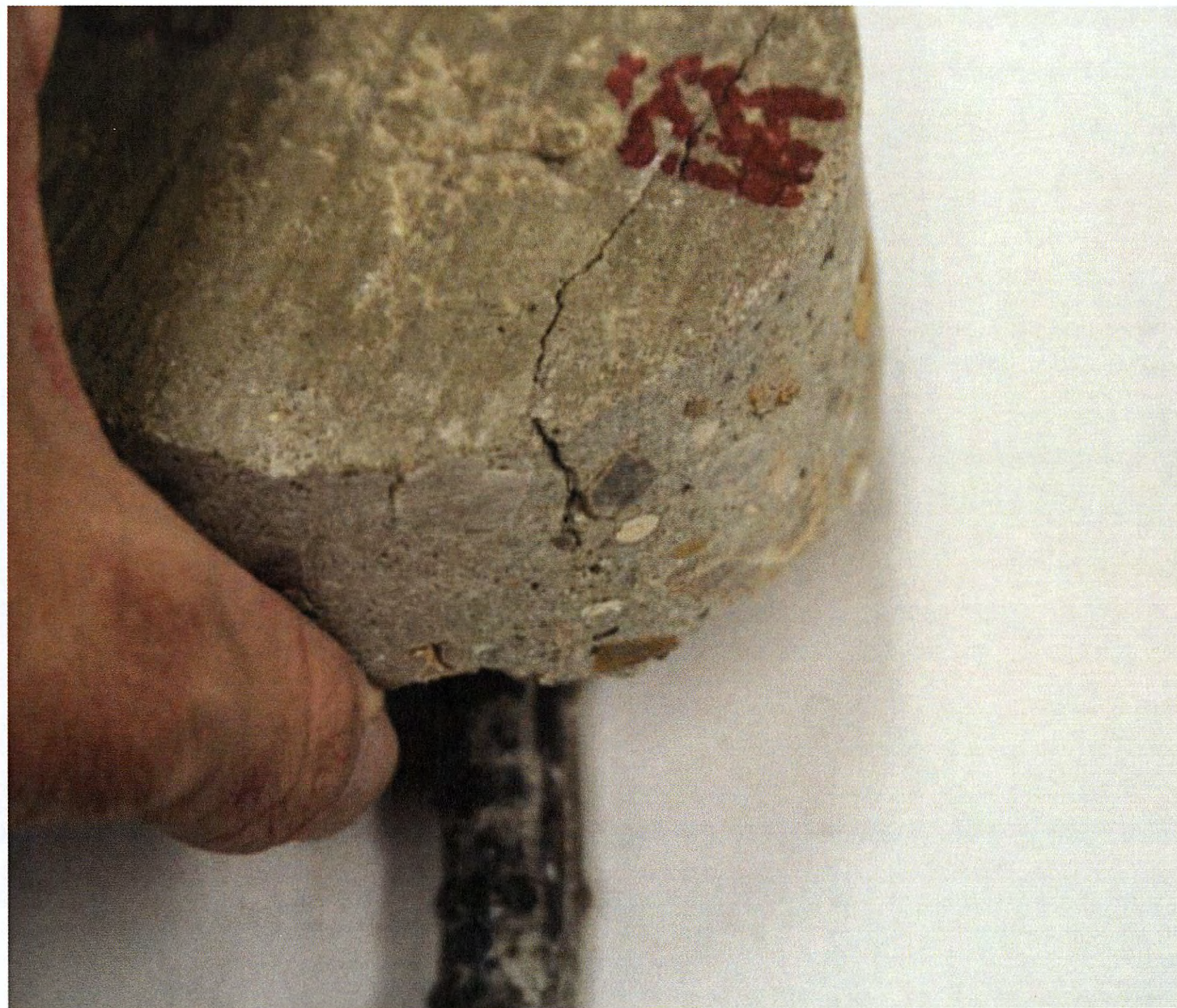
Figure 3-30. Core Extracted above Hoop with Surface Cracking.
