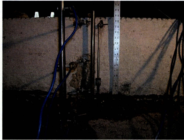
(a) Crackmeter for vertical movement measurements
