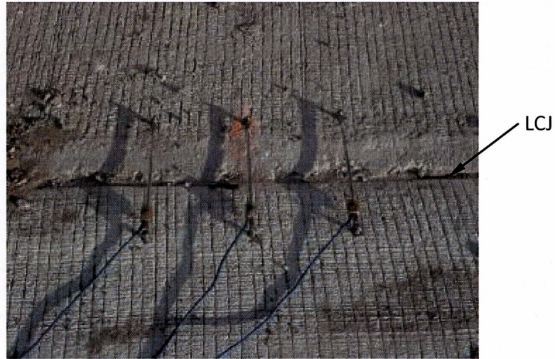
(a) Crackmeters installed at the surface across the LCJ in the tied section
