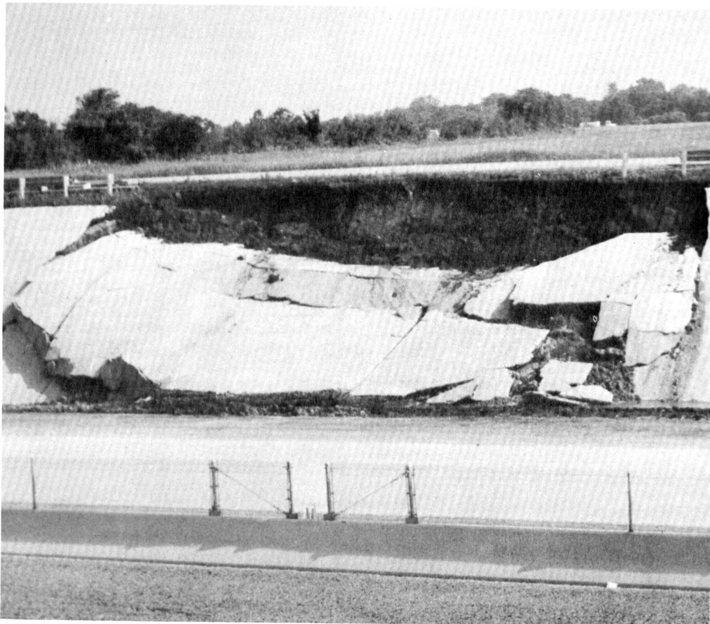
Figure 6.—Damage to highway embankment because of soil slippage in an area of Fairlie and Houston Black clays, 1 to 3 percent slopes.
